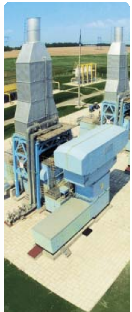
Gas compressor station in Tarutino (Ukraine). BSTDB financed, in two stages, a total of 18 million US dollars of the Trans-Balkan gas pipeline project bringing Russian gas through Ukraine to Romania, Bulgaria, Greece and Turkey.
